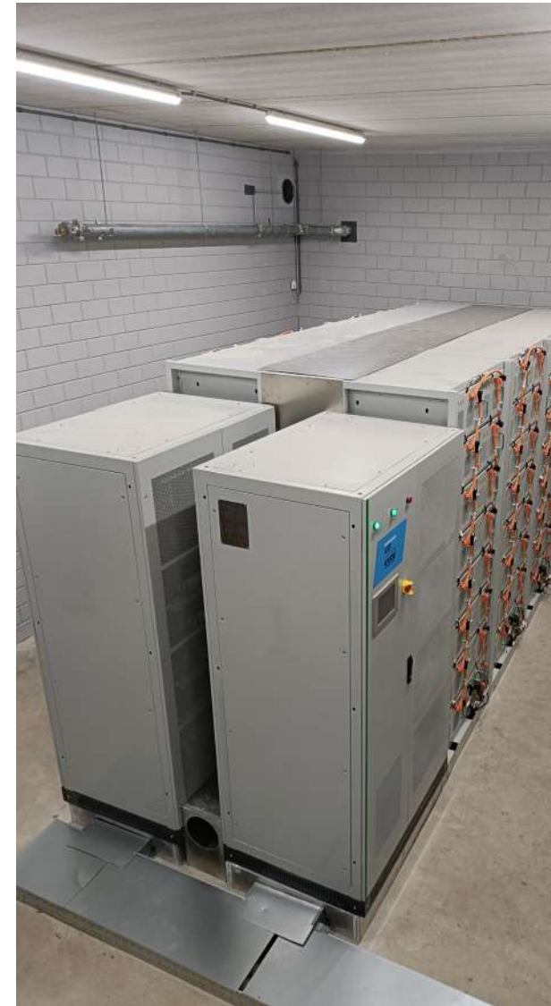
Battery system of Republica in Amsterdam related to the Atelier project. © Han Vandevyvere
